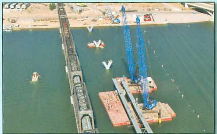
Figure 8: Aerial view looking north as cranes on barges proceed with bridge construction
