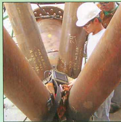
Figure 4: A certified inspector checks out full penetration welds of diagonals on bottom-pipe saddle while the welder looks on
