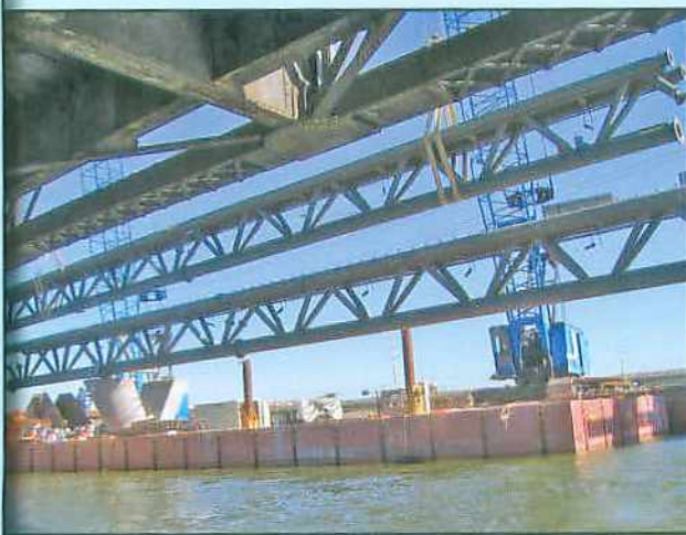
Figure 6: Two cranes on barges lift spliced truss segment into place on pier
